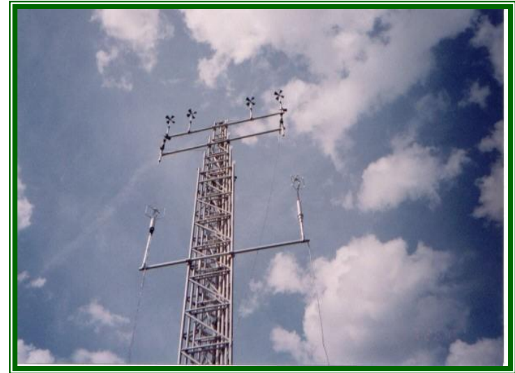
Anemometers Deployed on 30-Meter Crank-Up Tower
